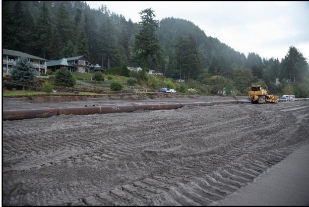
The pipeline that carried the dredged material is shown along with the newly created shoreline.
