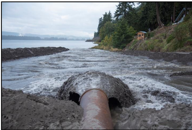
The sediment exiting the pipeline.
